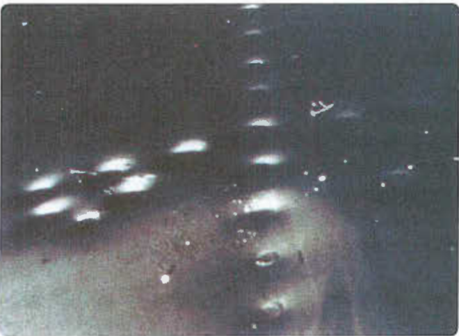
Figure 4-24. Skin bulging around fasteners.
