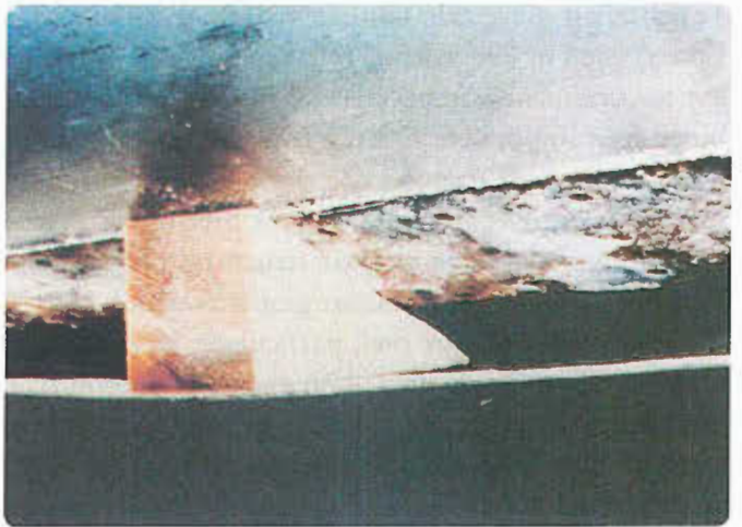
Figure 4-26. Close-up view of a corroded lap joint.
