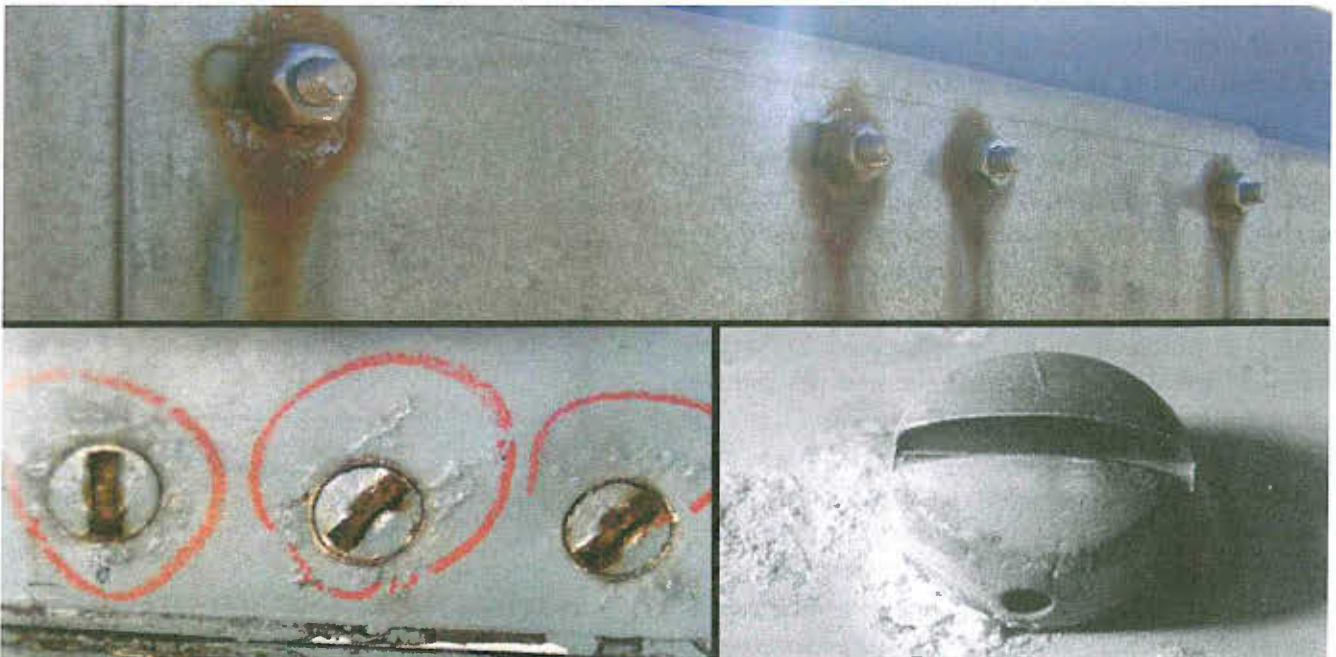
Figure 4-17. Corrosion around fasteners due to dissimilar metal contact.
