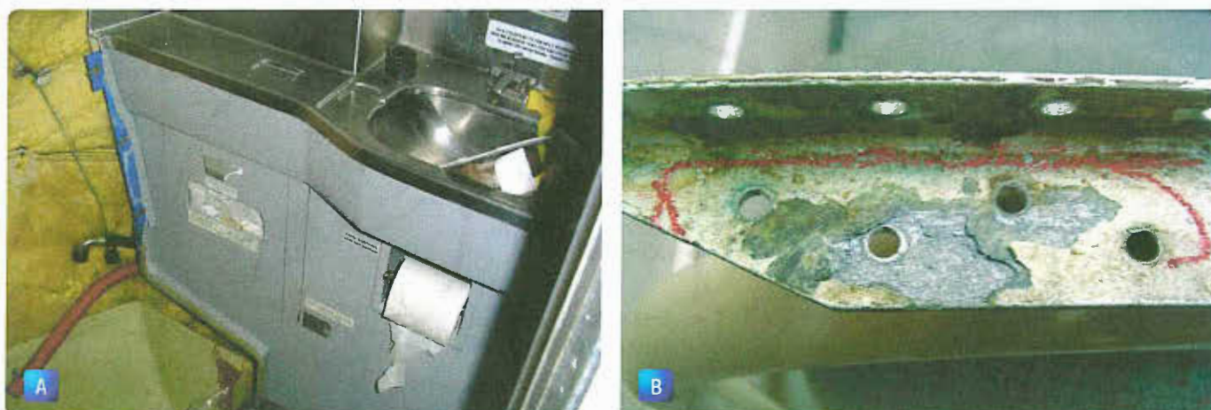
Figure 4-15. (A) Typical lavatory floor damages shown with the toilet is removed. (B) Corrosion caused by water and urine collecting on a lavatory attach bracket.
