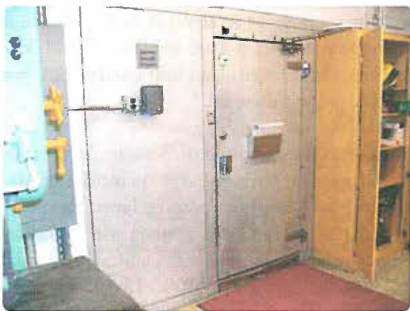
Figure 3-46. Walk-in freezer for storing prepreg materials.
