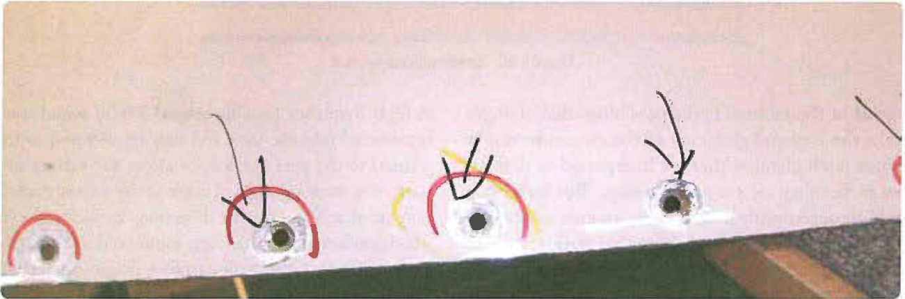
Figure 3-25. Corrosion of aluminum lightning protection mesh.
